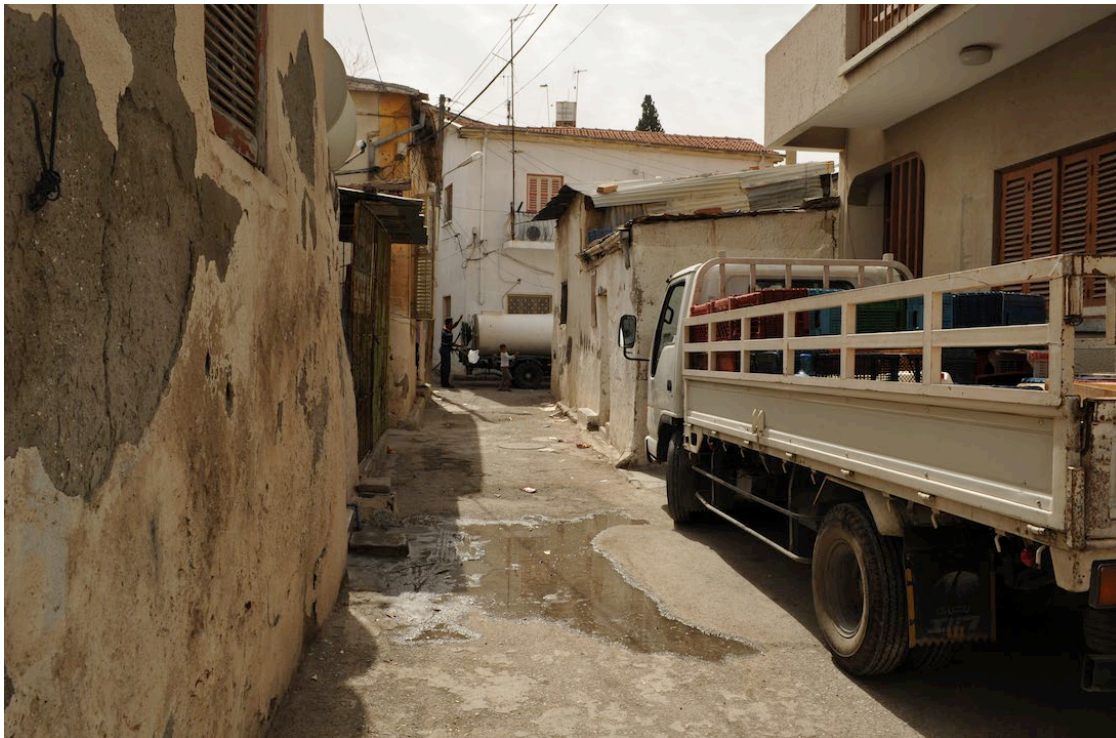
Figure 46 - Unrepaired damage to houses (shutters, windows, roofs) in Arabahmet neighbourhood within northern part of Nicosia Walled City (Photo credit: © Mohsen Shojaee Far, 2010).
